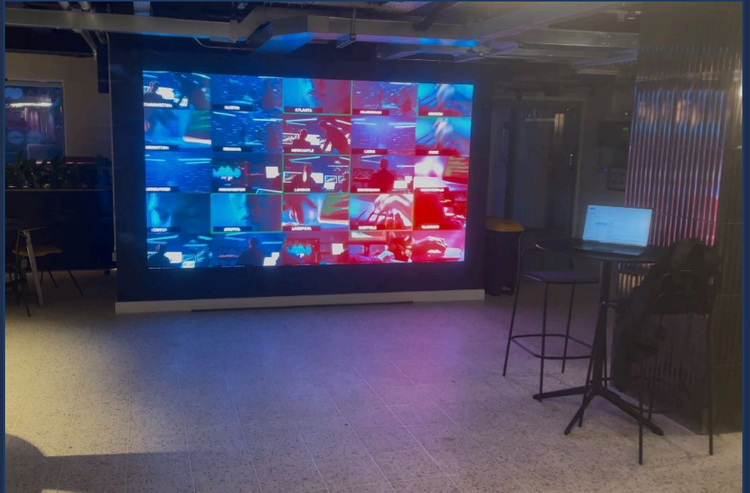
136" LG LED Video Wall serving as the visual centrepiece of the Ground Floor Presentation Space.
